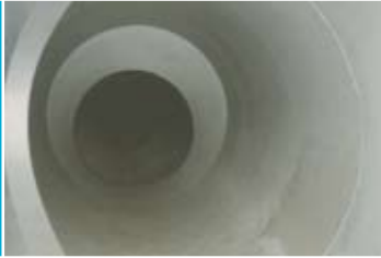
Internal Circle Water Pipe
