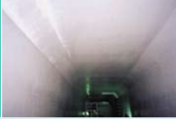
Internal Condensed Cooling Water Conduit
